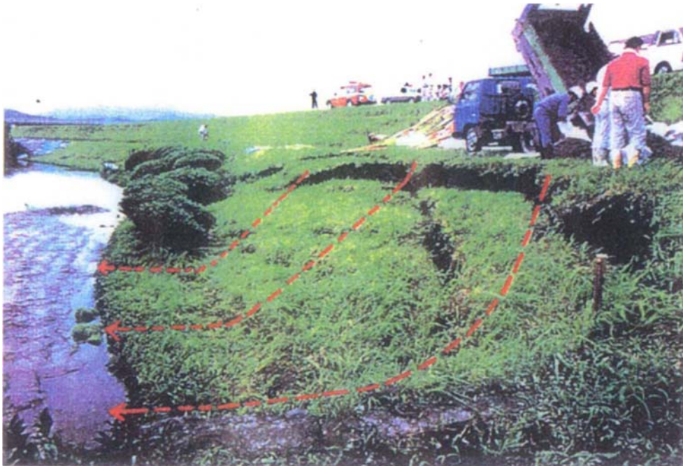
The slip failure induced by infiltration
