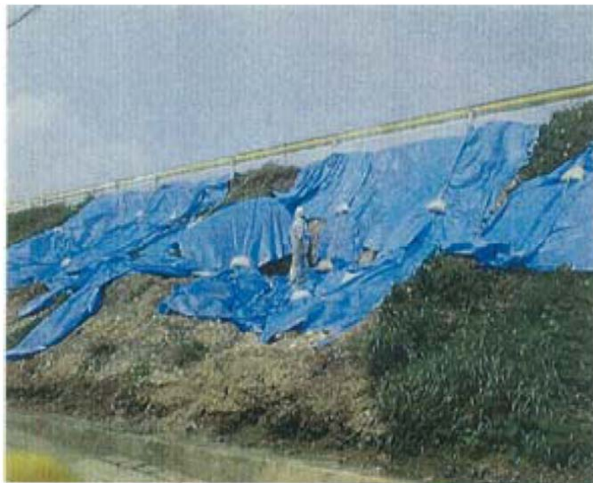
Figure 1-10 the infiltration failure in Shounaigawa River in Aichi, 2000 [9]
