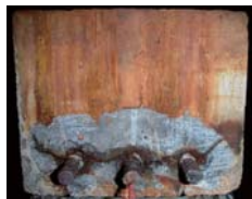
Fig. 8 Typical corrosion crack pattern on the end (F0-J0-20B)
